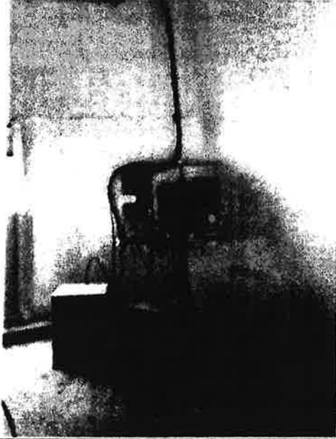
Equipment Inside the Water Tower
